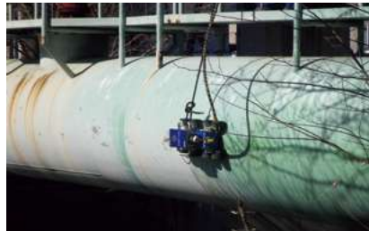
Ultrasonic thickness measurement
