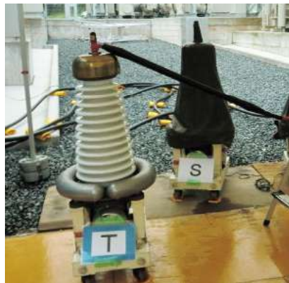
Withstand voltage testing
